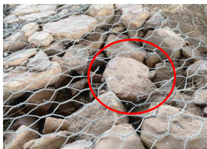
Damage to wire mesh of gabion in the bank protection work (source: Field survey)
