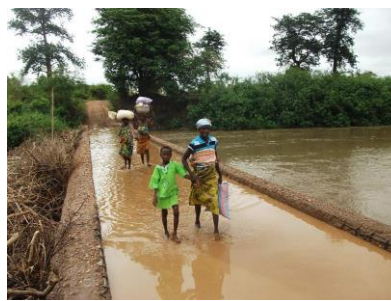
Residents crossing a sunken bridge on the Kara River in the early rainy season before project implementation (source: Preparatory Survey Report)
