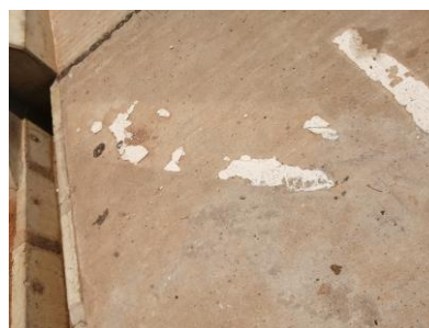
Road surface markings are detached (source: Field survey)
