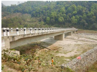
Photo 5: Daraudi Khola Bridge (At the time of the post-evaluation, source: external evaluator)
