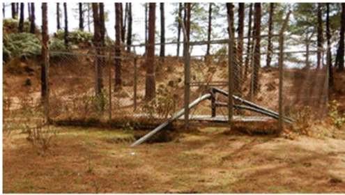
Photo 3: Chitre pressure breaking chamber (At the time of the post-evaluation, source: external evaluator)
