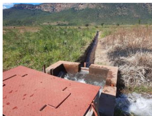
New irrigation facility in Block A (source: Evaluator)
