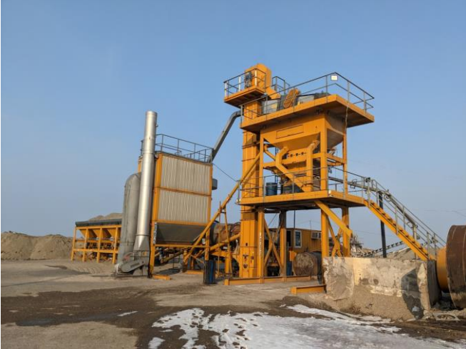
Asphalt plant installed in this project (Source: Photo taken by the External Evaluator)
