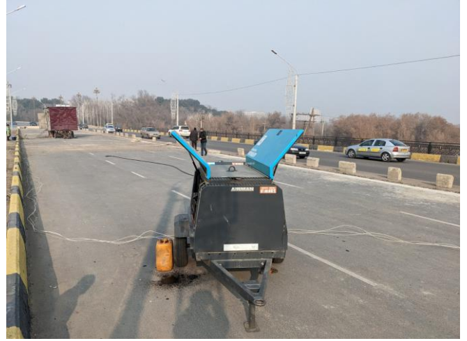
Compressor being utilised on a bridge (Source: Photo taken by the External Evaluator)
