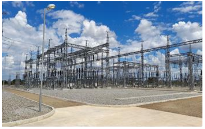
Project for Reinforcement of Transmission Network in Nacala Corridor assisted by JICA (2013-2018) (Namialo substation)
