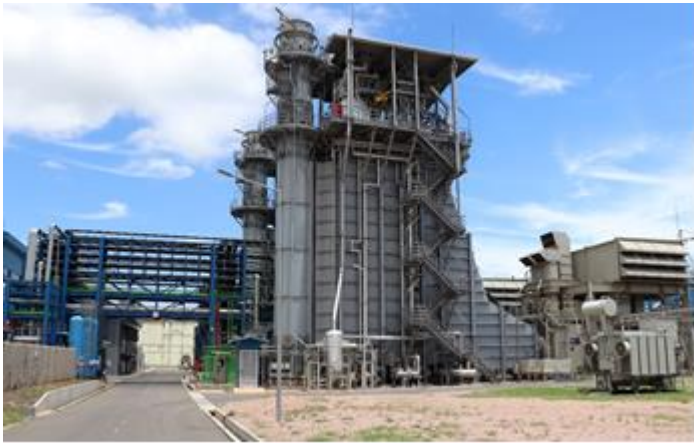
Maputo Gas Fired Combined Cycle Power Plant Development Project assisted by JICA (2013-2023)
