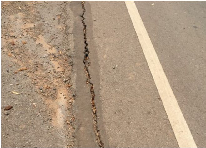
The Crack of Approach Road (Xe Tha Mouak Bridge)
