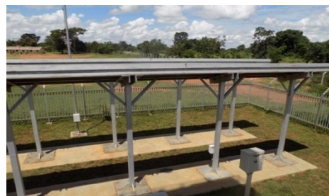
Solar Power Generation Facility (Buseta)
