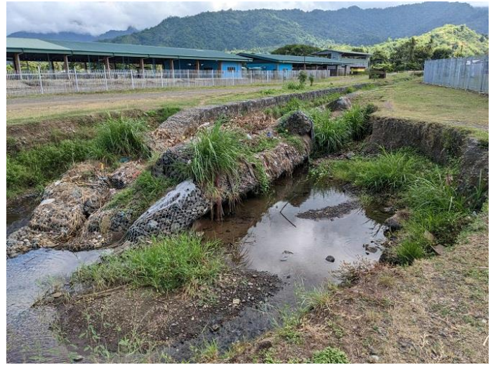
Small Creek Eroded by Heavy Rainfall (Source: External Evaluator)
