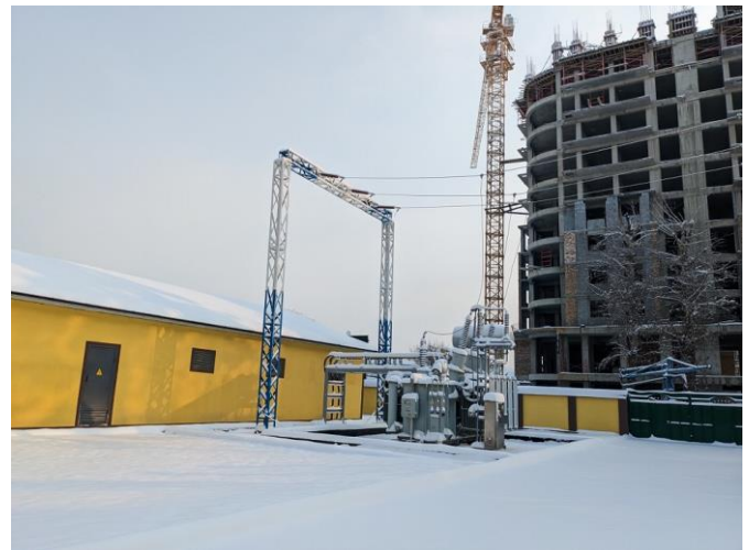
Small-scale substation independently developed by the executing agency after the project (Source: External Evaluator)
