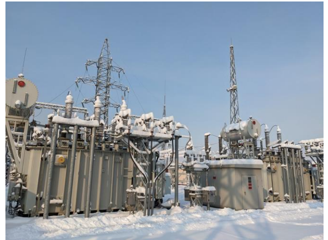
Radiostantsiya Substation Developed Under the Project
