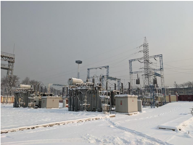
Substation equipment developed at the Promyshlennaya Substation (Source: External Evaluator)
