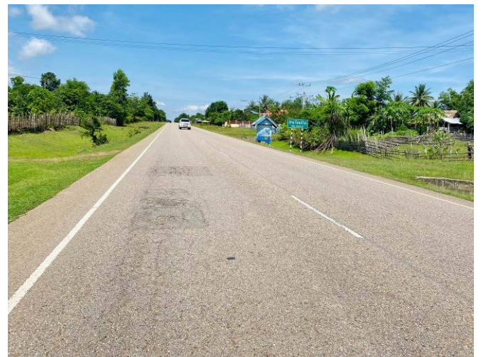
A section of National Road No. 9 which is maintained annually after the support by the project
