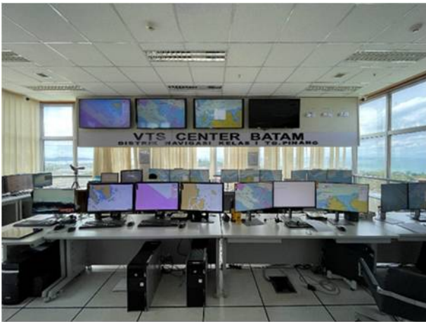
VTS Batam Control Room
