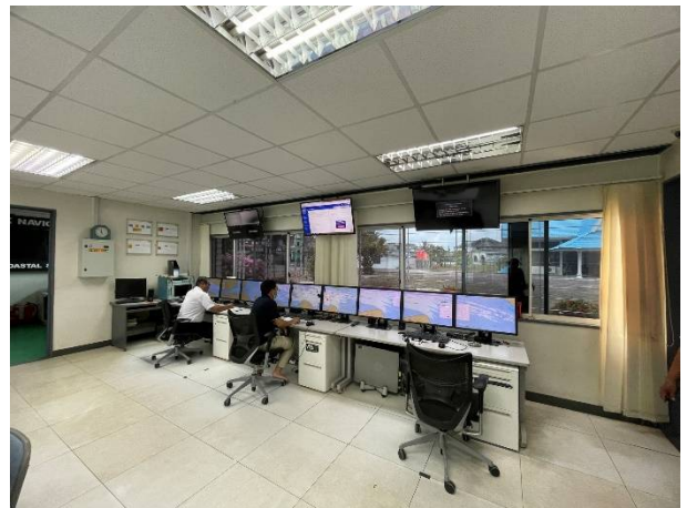
VTS Dumai Control Room
