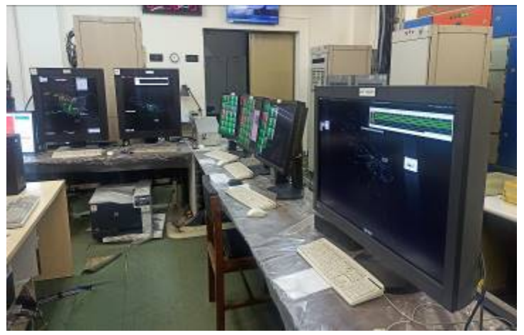
This project strengthened the Surveillance System procured under the Grant Aid “TIA Modernization Project”, which is used to provide ERCS.
