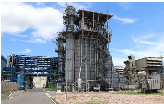
Belem substation (440 kV) in Huambo Province started its operation in 2019
