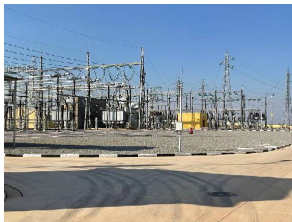
Belem substation (440 kV) in Huambo Province started its operation in 2019
