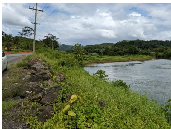
Scoured Point of a River Restored with the Project Fund (Source: External Evaluator)
