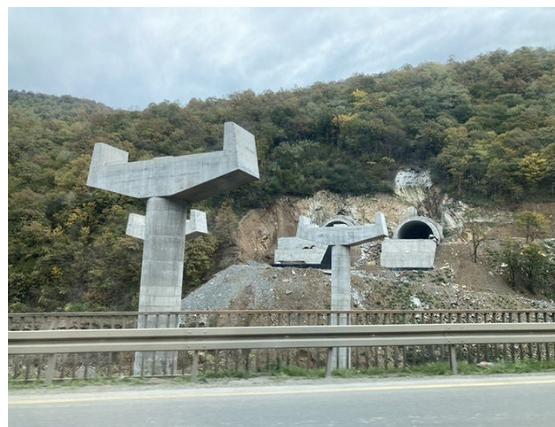
Photograph 4: Construction Work Between Shorapani and Argveta on the East Side of Zestafoni
