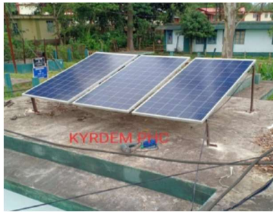
Solar panels installed at a primary health center
