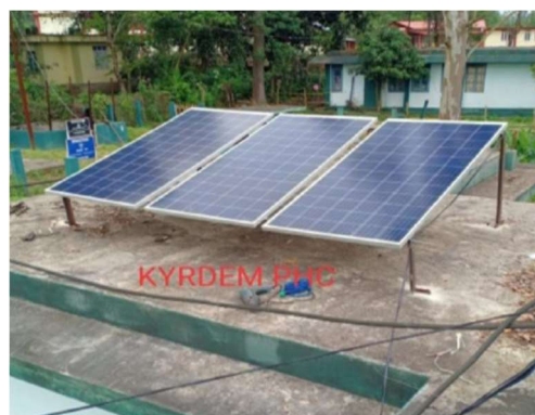
Solar panels installed at a primary health center (Source: NITI Aayog)
