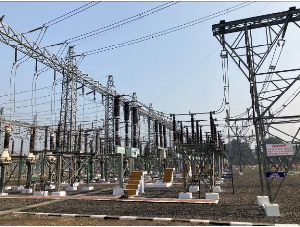
Switch-yard of substation (Jabalpur substation: photo by the external evaluator)
