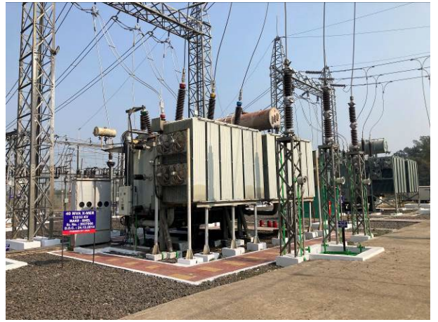
Transformer of the Project (front), transformer added later (rear) (Jabalpur substation: photo by the external evaluator)
