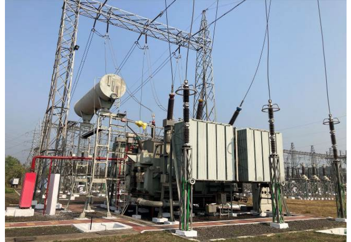
Jabalpur Substation constructed under the Project (Source: photo by the external evaluator)
