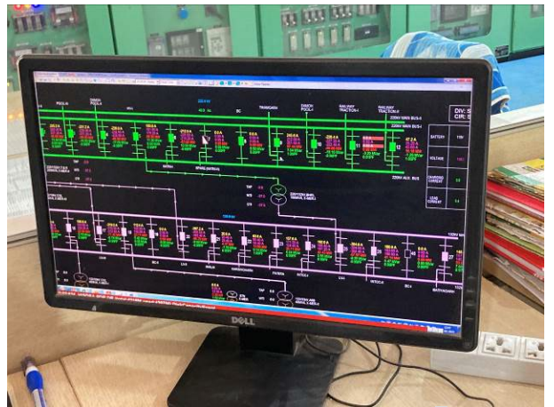
SCADA display at substation (Damoh substation: photo by the external evaluator)
