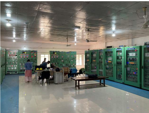
Control room of substation (Damoh substation: photo by the external evaluator)
