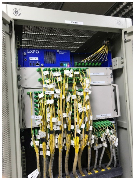
Photo 2: FMS procured under the project (Source: Ex-post evaluation team)
