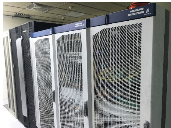
Photo 1: Telecommunication equipment storage cabinet at the Al-Mamoon site (Source: ex-post evaluation team 1 )
