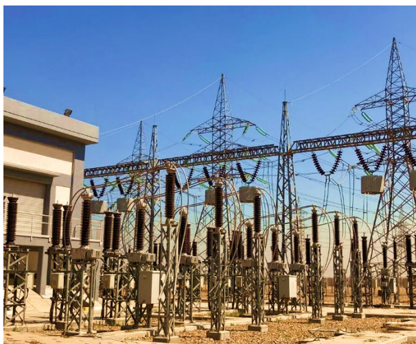
Newly constructed substation (suburb of Baghdad) 1
