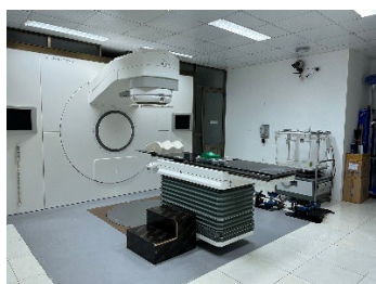
Image 2: Radiotherapy equipment installed at C Da Nang Central General Hospital
