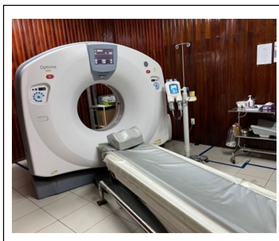
Image 1: CT scanner (source: taken by the evaluator)
