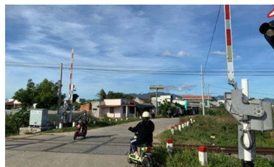
Image 3: Improved level crossing (ancillary facility of Song Quao Bridge in Ninh Thuan Province) (source: Photographed by the ex-post evaluator)
