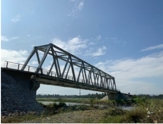
Image 5: Gia Huu Bridge in Binh Dinh Province. Completed in 2021, the bridge was constructed using technology from this project and government funding after the project's completion. (source: Photographed by the ex-post evaluator)
