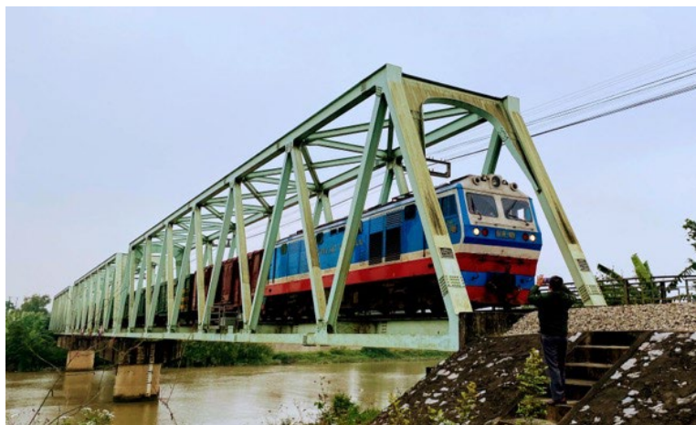
Image 1: Do Len Bridge in Thanh Hoa Province (source: Photographed by the ex-post evaluator)
