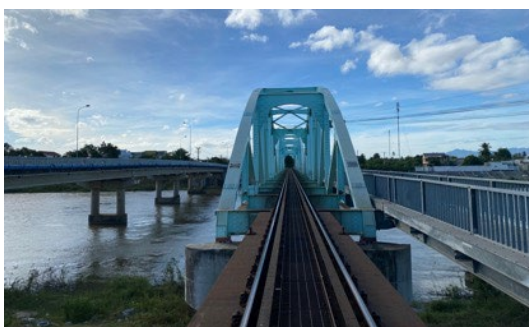
Image 2: Thap Cham Bridge and its side road in Ninh Thuan Province. The bridge used Japanese technology such as directly fastened track. (source: Photographed by the ex-post evaluator)
