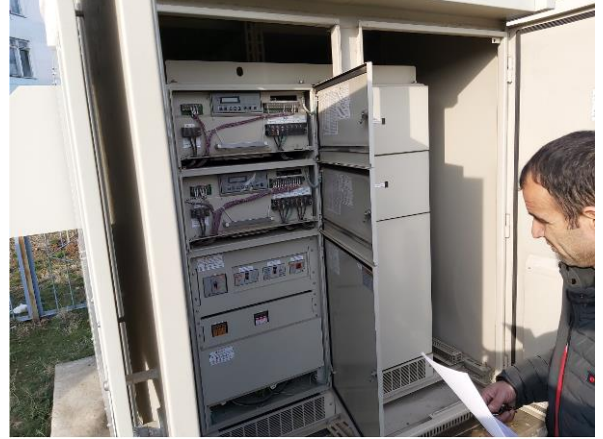
Control Panel of National Medical Center Shifobakhsh
