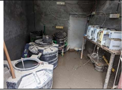
Hydrogen Gas Generator, Jwagal LCD, being damaged due to inundation from flooding
