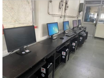
SCADA Control Center.
