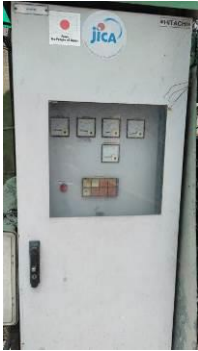
Control Panel at Pilot Project Site in Pitampura.
