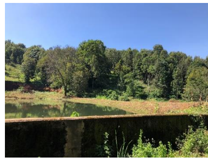
Photo 4 Irrigation facilities with uncompleted construction: Orumwi Irrigation Scheme in Kilimanjaro Region (Photo taken by the evaluator)
