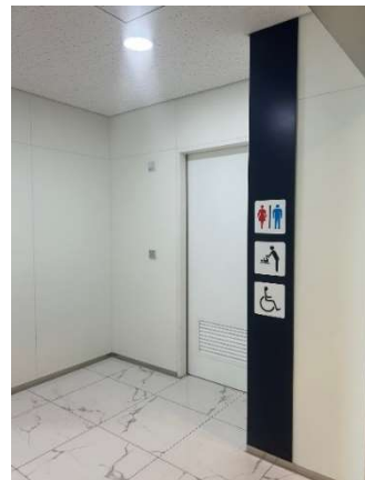
Photo 5 Installed Multipurpose Toilet
