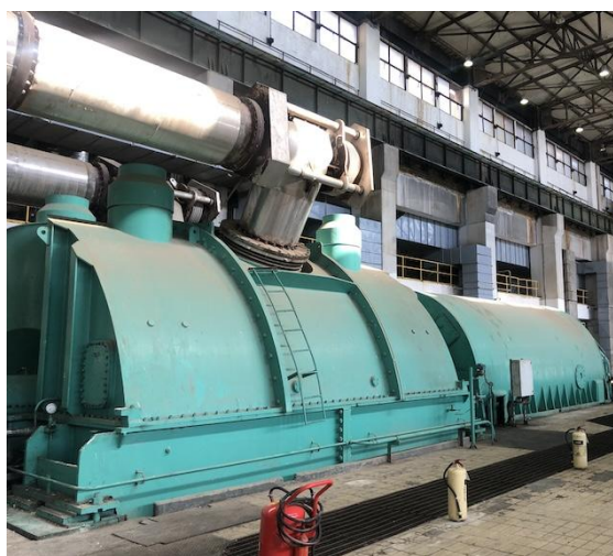
Image 3: Unit 3 turbine-generator (source: Photographed by field survey assistants)
