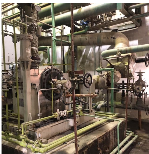
Image 2: Unit 3 boiler equipment (source: Photographed by field survey assistants)
