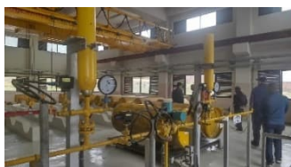
Photo 1 Chlorine Disinfection Injection Facility
