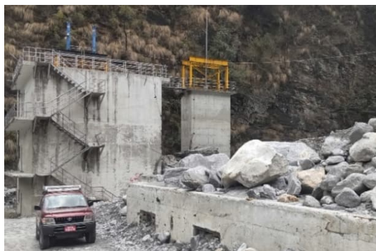
Photo 7 Part of water intake facility buried by mudslide
