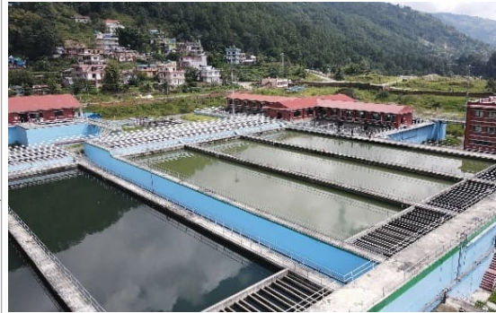
New Sundarijal Water Treatment Plant (source: Implementing Agency)
