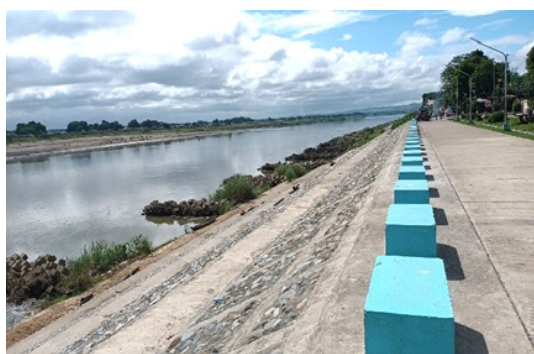
Photo 1: Revetment and Spur Dikes Constructed as Part of the Cagayan River Sub-Project
