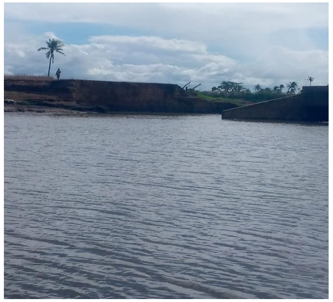
Protective Dike destroyed during the natural Disaster. (Edson Marina)
