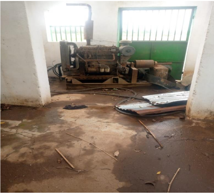
Irrigation Pump not working after the natural disaster (Edson Marina)
