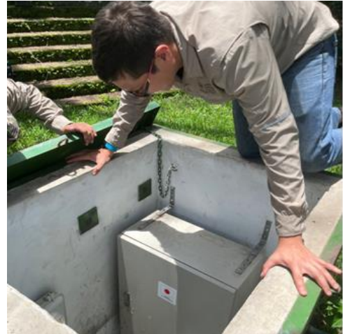
MARN engineering and maintenance unit team inspecting the equipment procured by the project during field visits in the ex-post evaluation.
