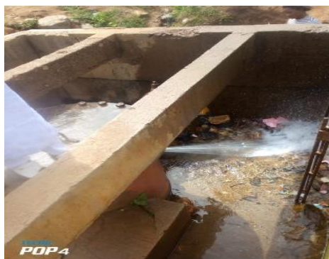
3. First location of detected leakage at Apo district
