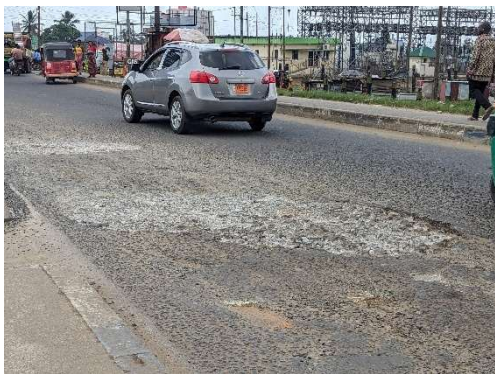
Photo 13: Potholes just before the Jamaica Road junction on Phase 1 road (November 2024) (Source: Evaluator)
