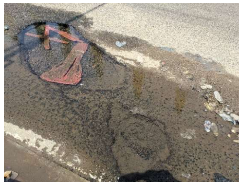
Photo 14: Potholes caused by leaks from sewer pipes (November 2024). Liberia Water and Sewer Authority repaired the leakage in March 2025. (Source: Evaluator)
