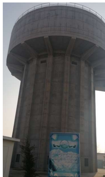
Elevated Tank Installed in This Project (Source: Photo taken by the local consultant)
