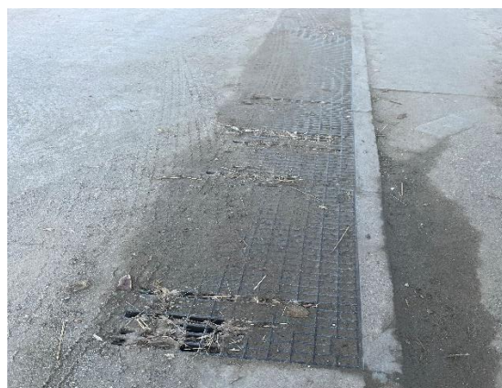
Photo 6: Clogged roadside ditch (Source: Photo taken by the external evaluator)
