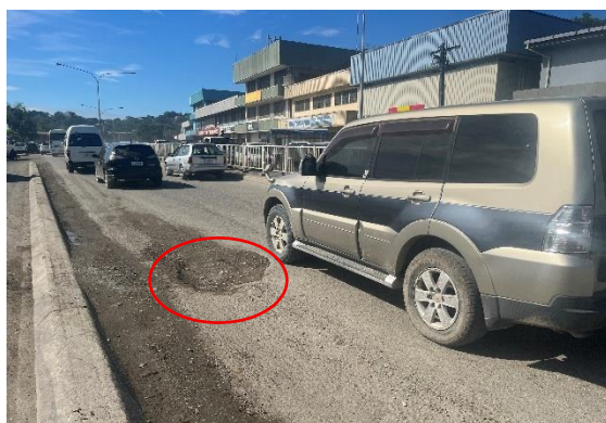
Photo 3: Condition of road deterioration in front of the Central Market (red circle indicates deteriorated road surface) (Source: Photo taken by the external evaluator)
