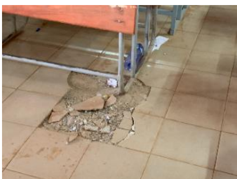
Photo 13: Floor tiles peeling off in the classroom
