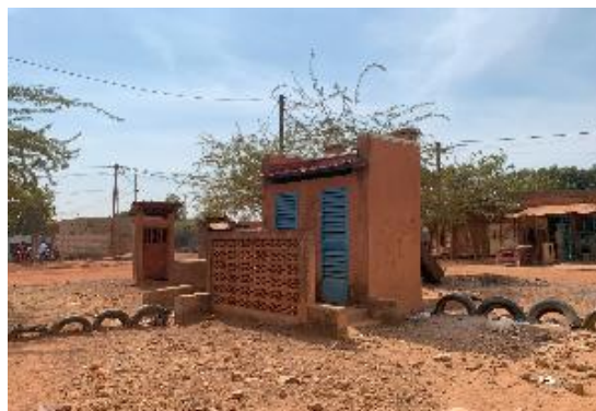
Photo 12: A-02: Somgande B, D, where no wall surrounding the school (The toilets are located right next to the road. Additionally, tires have been laid out to prevent vehicles such as motorcycles from entering the school grounds.)
