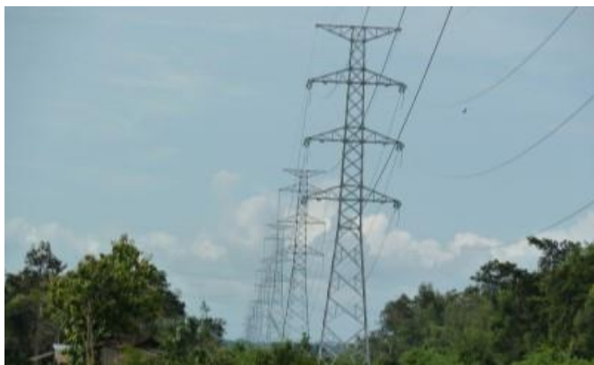
230 kv power transmission line from Hinherb Substation to Naxaythong substation.
