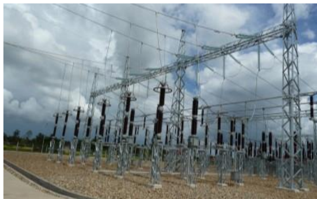
230/115 Kv Power Substation at HinHerb district
