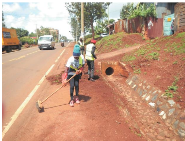
Cleaning the road drainage by a female worker (Photo taken by JICA expert)
