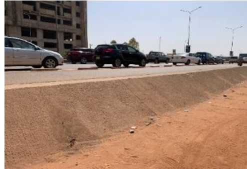
Photo 1: Section with a Height Difference Between the Road and the Sidewalk Source: Taken by the evaluator
