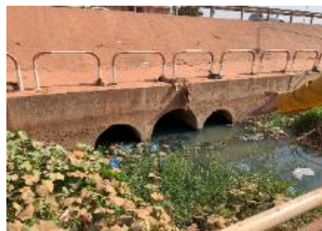
Photo 4: Sediment Accumulation Observed at the Outlet of the Cross Drain (Source: Taken by the evaluator)
