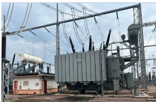
Photo 2 Infulene Substation T2 transformer (Source: taken by the external evaluator)
