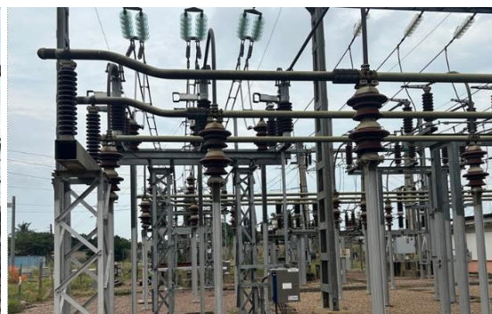
Photo 3 Infulene Substation 66 kV disconnecting switch (Source: taken by the external evaluator)
