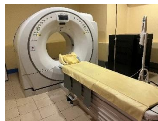
Photo 3. CT Scanner Installed at Champasak Provincial Hospital
