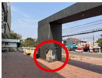
Photo 10. ER Entrance of Setthathirath Hospital (damaged by a hospital user's vehicle and left unrepaired)
