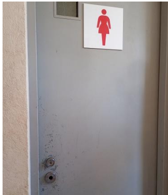
Photo 6: The Patient Toilet at Gulu RRH with a Missing Doorknob (source: taken by the evaluator)
