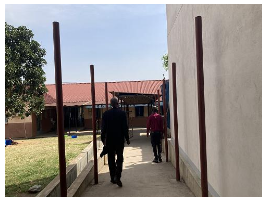
Photo 2: The Walkway at Arua RRH with an Unfinished Roof (source: taken by the evaluator)
