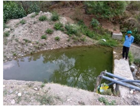
Photo 8: Silt Accumulation at the Weir in a Lift Irrigation Area in Kangra District (Although countermeasures had been taken by the KVA in the past, siltation continues.) (Source: Taken by Evaluator)
