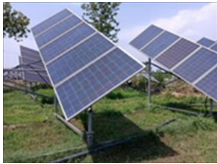
Photo 7: Solar Panels in Una District (Source: Taken by Evaluator)
