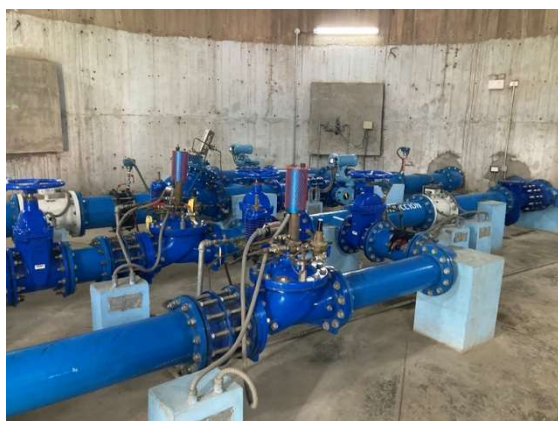
Photo 1. Valves in a water distribution reservoir
