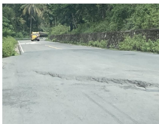
Photo 5: Section of the Manatuto-Baucau Road with Surface Unevenness (Source: Taken by the evaluator)
