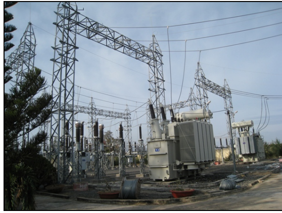
Photo 4: Phan Ri substation
