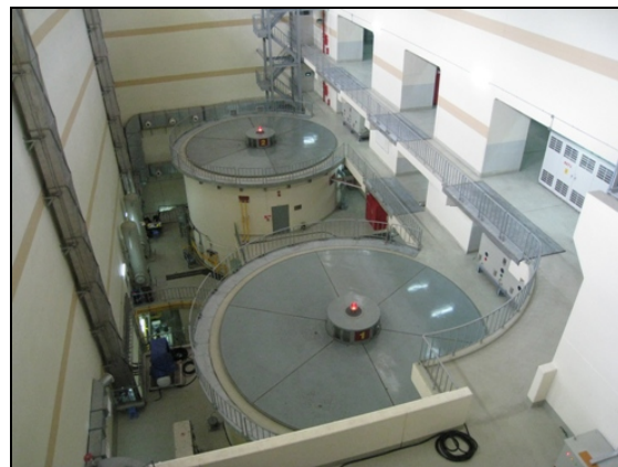
Photo 2: Hydropower plants with 300MW (150MW x 2)
