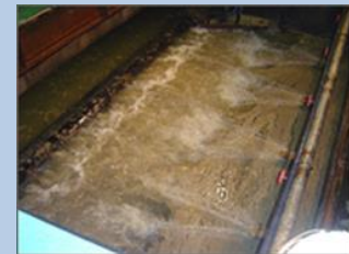
Example of scum removal equipment with low electricity consumption.
