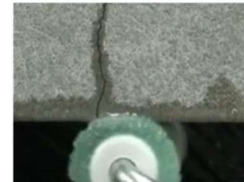
Penetrates into cracks on ceiling
