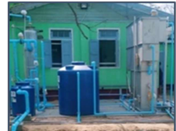
Water Purification Equipment (Fiber Filtration System)
