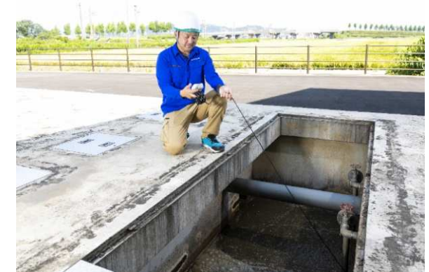
Settlement Drainage System
